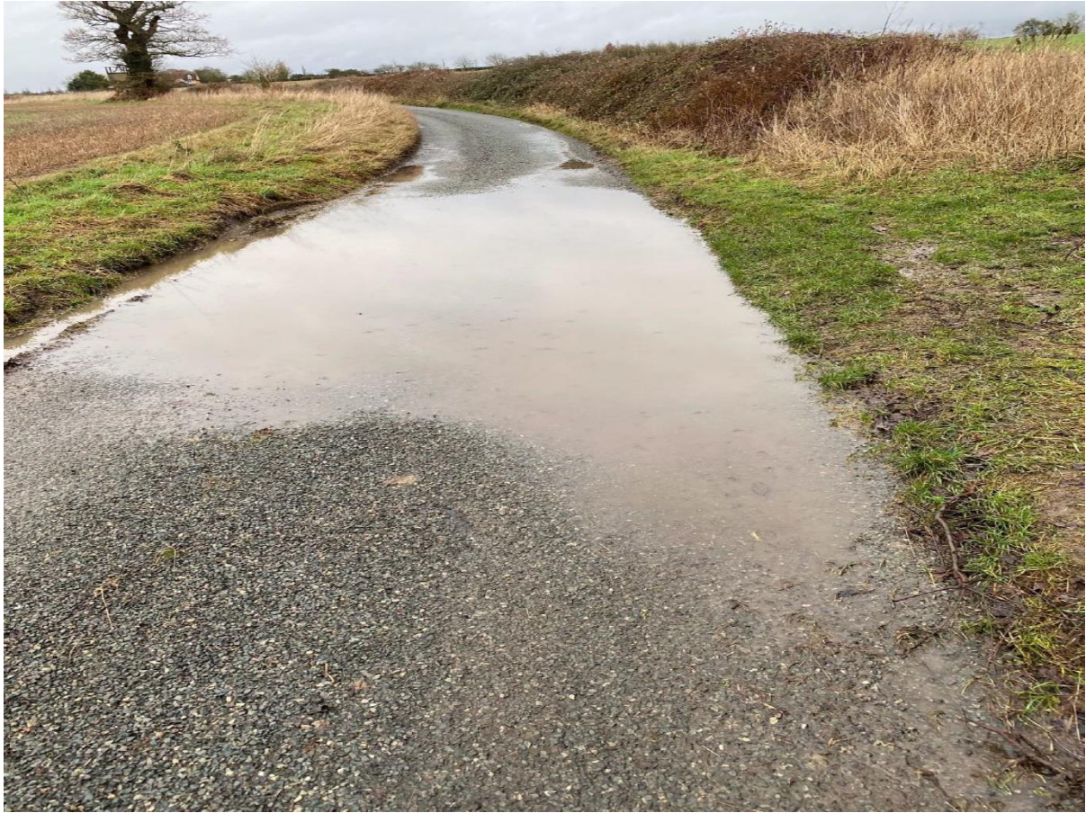
Image8—Looking away from Stanstead—road often floods at this point
